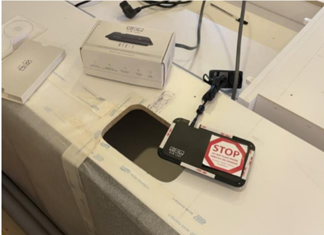
1. Cut hole in island carcass - ensure the opening is big enough to be able to remove charger if needed
