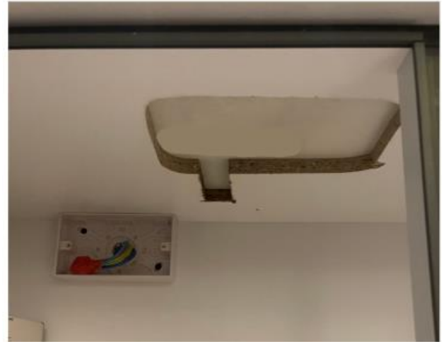
2. Ensure power is available to charger either in the island or cupboard.
